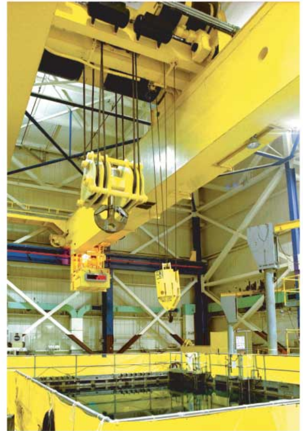
150 Ton Nuclear Fuel Handling Crane
